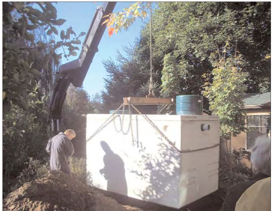
A five tonne water tank is lowered into the ground in Bill Bean's backyard. in Kitchener. It means they will have lots of water for gardening, even during droughts.
